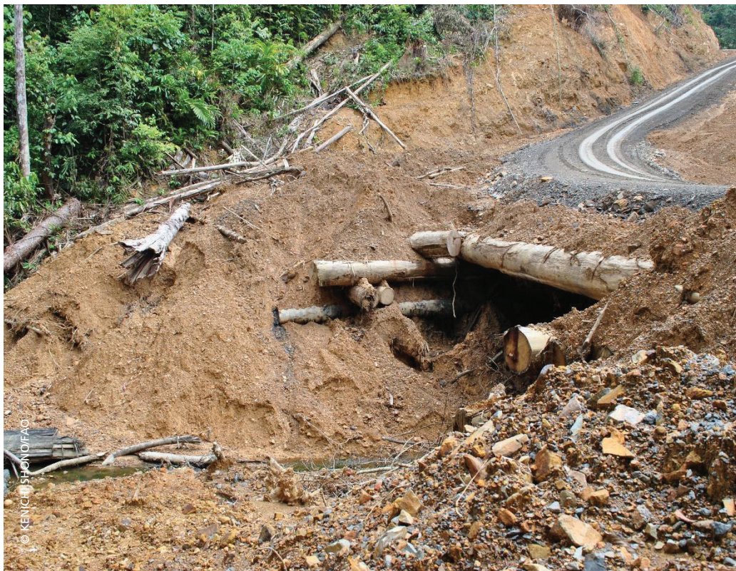
A logging road with an improperly constructed stream crossing
